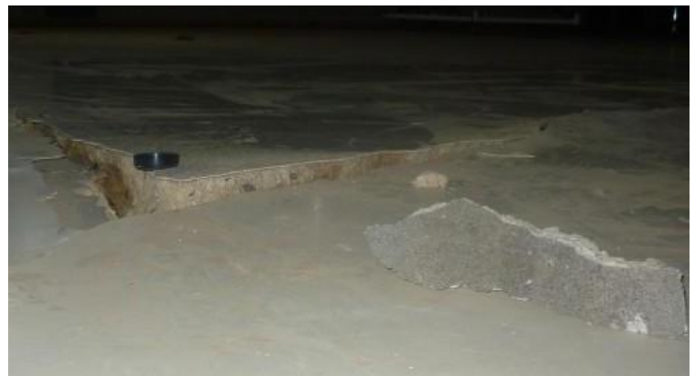
FIGURE No. 20: PAVING RAISED BY WATER UNDERGROUND
