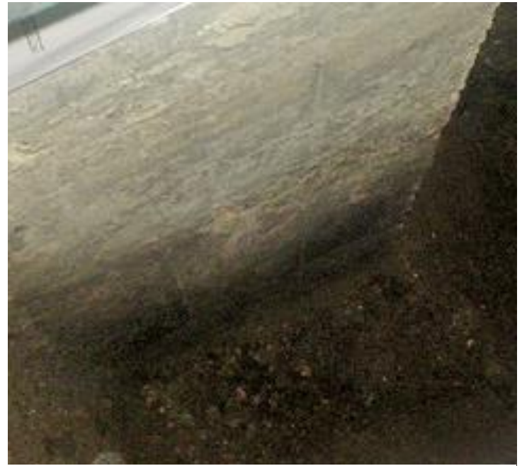
FIGURE No. 6: LOCALISED SURVEY TO DETERMINE THE NATURE AND DEPTH OF THE EXISTING FOUNDATIONS
