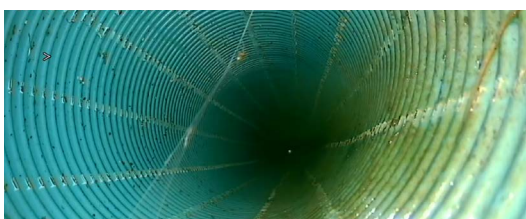
FIGURE 28: INTERIOR VIEW OF THE INFILTRATUBE
